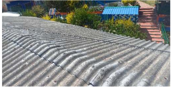
Roofing in need of replacement.
